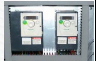
Two speed inverters
